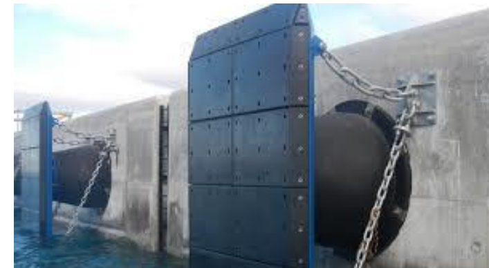
Maintenance Expenses Reduction
